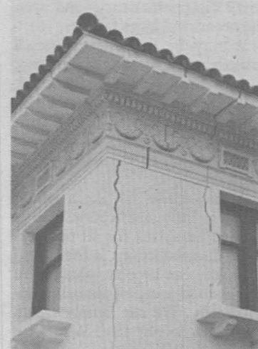
QUAKE DAMAGE—Ambassador Hall received structural damage in the June 28 quake. [Photo by Charles Feldbush]
